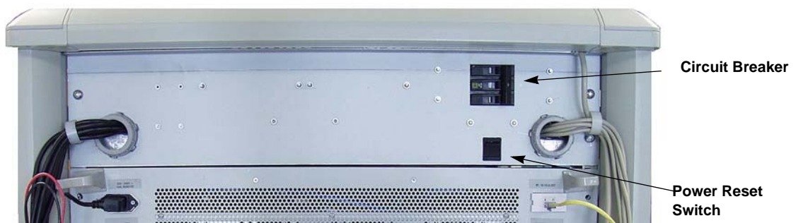
Figure 1.3 Upper Rear View of System Rack
